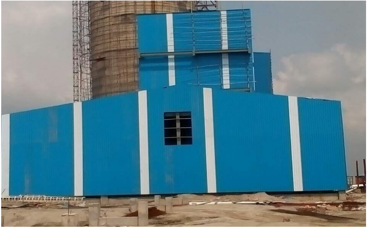
Bengal Cement-Packing Unit, Barodi, Narayangong.
